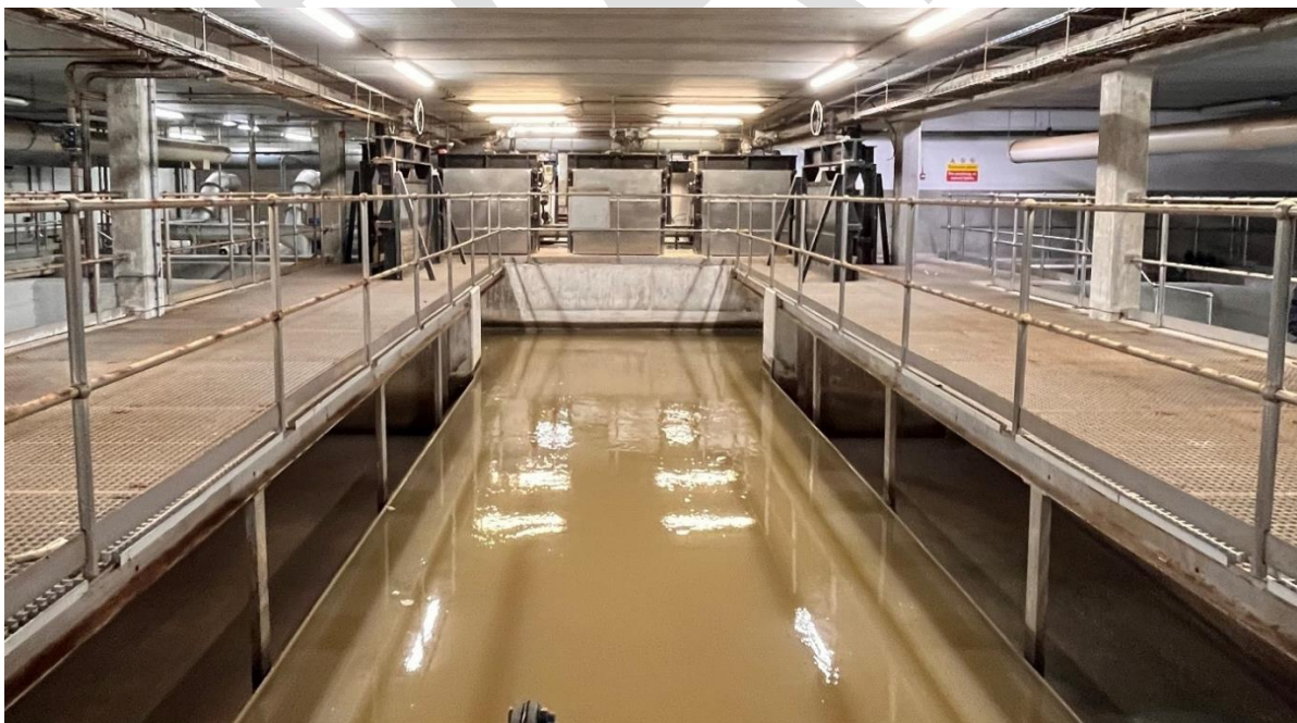
Figure 3-4: Mutton Island WWTP FFT Double Sided Weir
